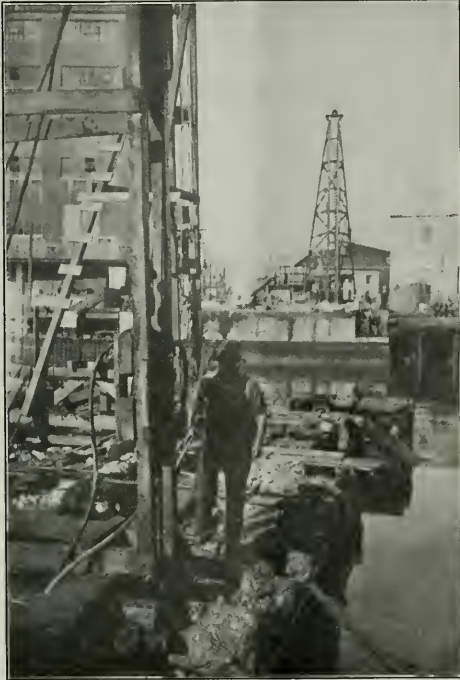
North Pier, Showing Steel Cut and Waiting to Be Removed. Note Corner of Eight-Story Southern Pacific Terminal Warehouse.
